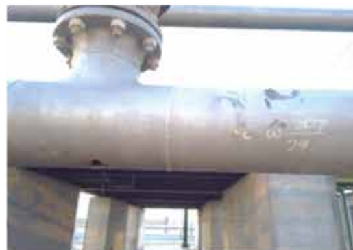
View of tee with through wall defect
