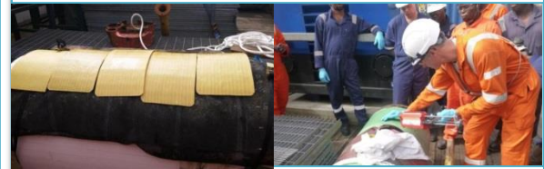
Composite plate manufacture on the foot print of the dented area & primer application (training picture).
