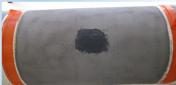
Fig. 2: View of the delimited repair area to be wrapped & Example of filler F3X8 application on 12" pipe defect
