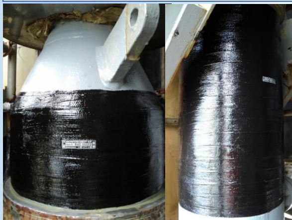
Figures 3 & 4: Composite wrappings finished on heat exchanger (2 defected areas)
