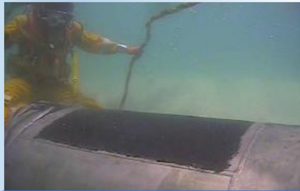
Figure 1: P3X30 primer application on defected area (step 2)
